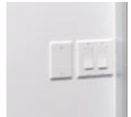
Final room controls were easily added to the installation.
